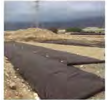
The chambers, covered with stone and geotextile, were installed beneath a baseball and small soccer field, beneath approximately 10 feet of cover. Photo: courtesy of CULTEC
