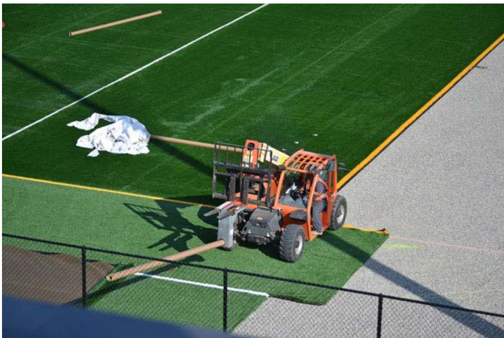
OHNO construction workers and FieldTurf Co. install the polyurethane grass and insert grass sections with colored lines that are sport specific. Photo credit: John Saringo-Rodriguez / Daily Sundial
